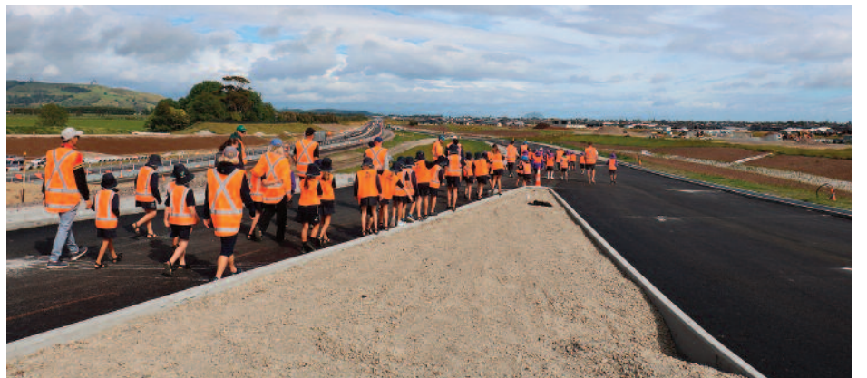
Children from Golden Sands School and Suzanne Aubert Catholic School enjoyed a visit to the interchange construction site.
